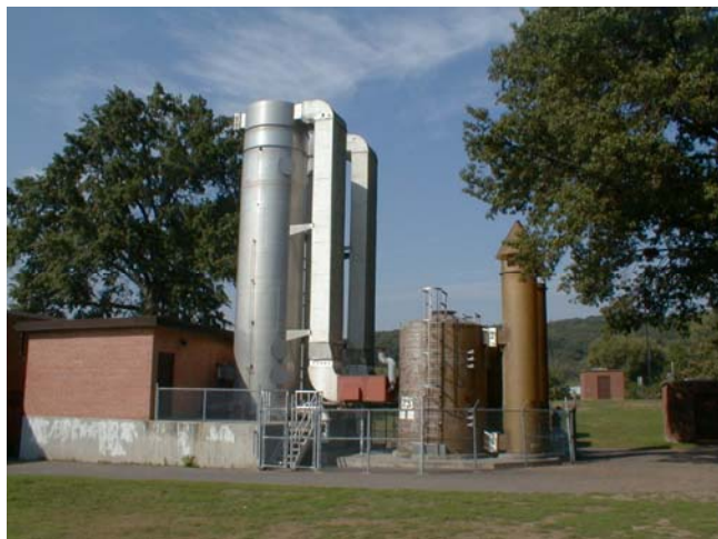
View of chemical air strippers attached to municipal wells at the Wagaraw site.
